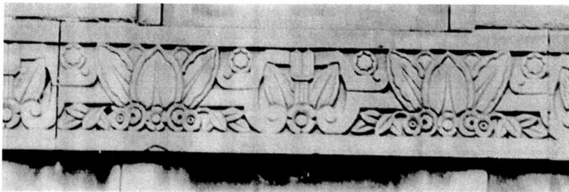
The West Town State Bank Building is an excellent example of the Art Deco architectural style. It has an angular, crisp-edged composition with a vertical emphasis, including a prominent penthouse tower facing Madison (top). Ornament consists of both geometric and foliate Art Deco-style detailing and abstracted Classical ornament, including pilasters and eagles.
